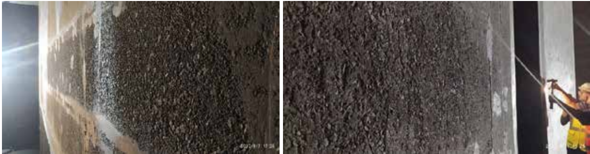
Figure 4: Severe abrasion in Unit 3 draft tube (left) and abrasion in Unit 3 spiral case(right)
