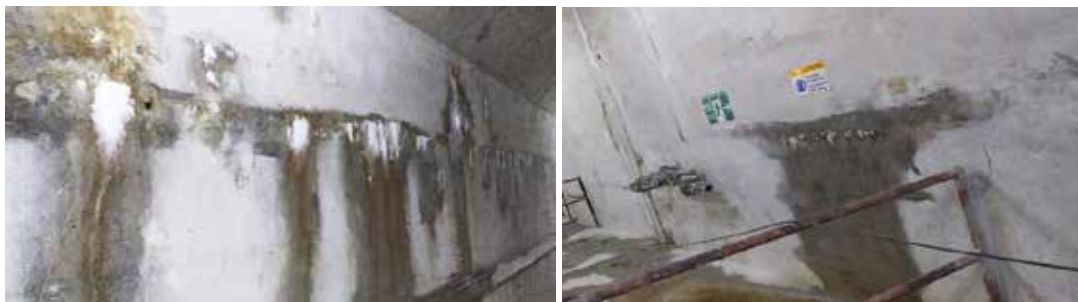
Figure 3: Damp spots and leakage along lift joints at EL1024 and EL1017
