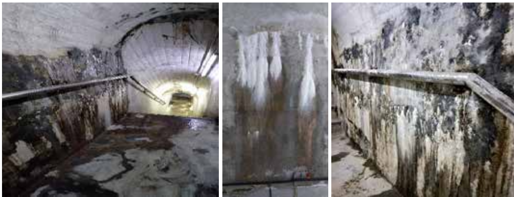
Figure 2: Concrete leakages along staircase from EL1025 and at EL1017
